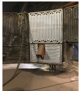
Injector installed on the water-cooled side wall of the furnace
